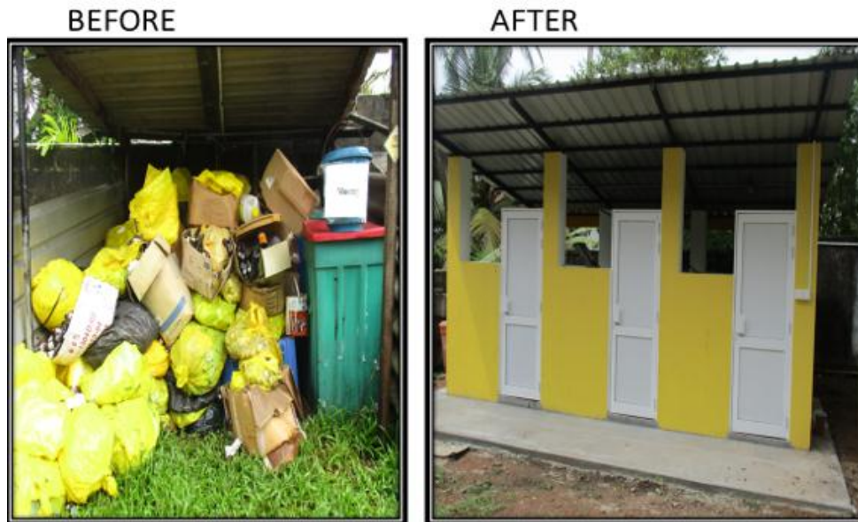
Newly built clinical waste store
